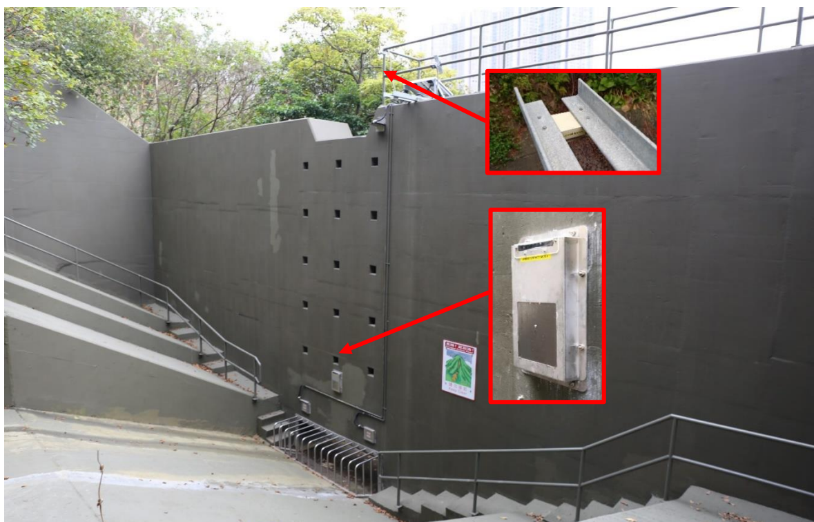
Pilot test of Landslide Detection System in Sham Tseng San Tsuen
