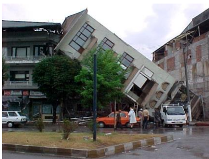
Tilted building due to liquefaction
