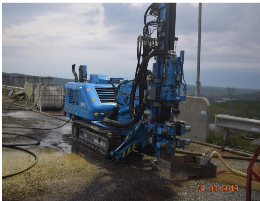
Figure 4: Drilling inside the tunnel and on the body of Mosul earth dam.
